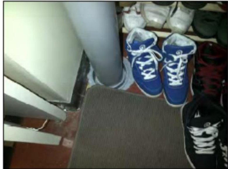
PHOTO 119 - UNIT G3 - SUCTION POINT
